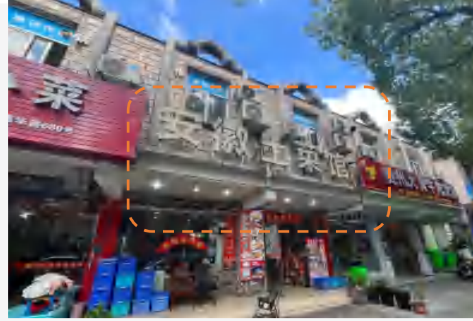
构件管线裸露
